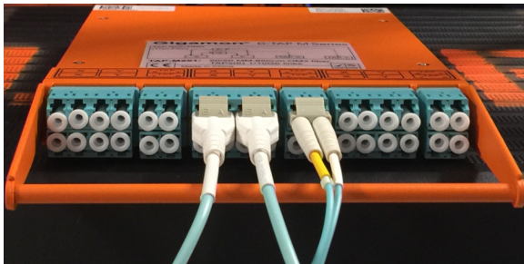
Figure 11 LC Connectors connected to TAP
